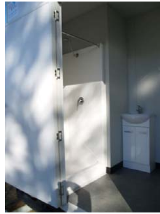
Inside: Shower Cubicle and Vanity
