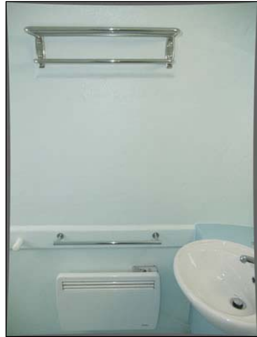
Panel Heater / Towel Rails / Vanity
